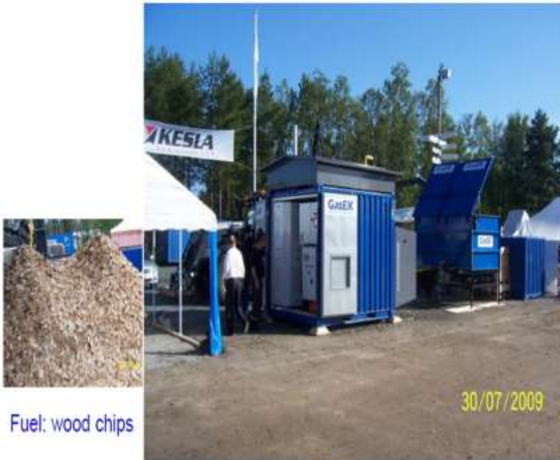
The 150kW wood gas container and wood chip storage
